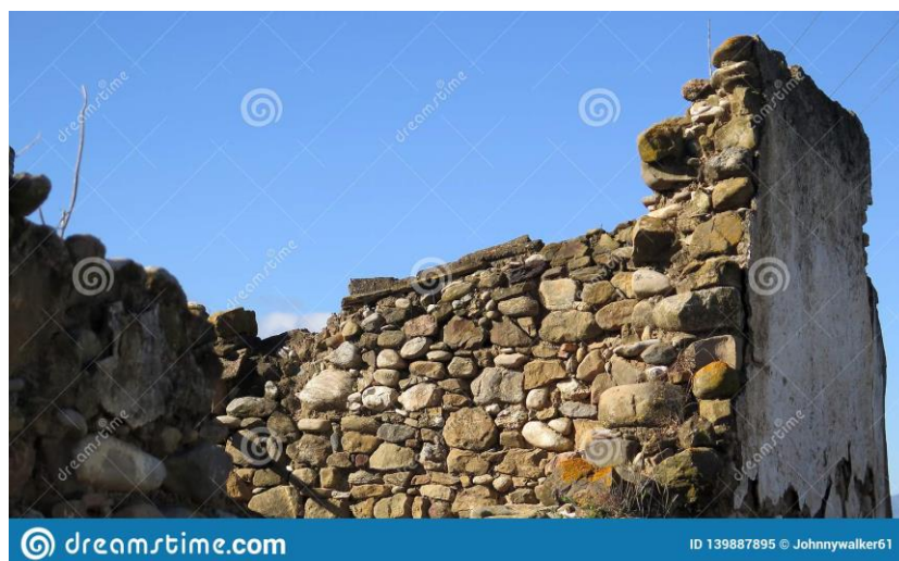
Figure 13 Broken Walls and Debris around the Level
