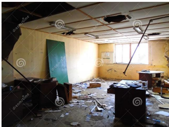
Figure 18 Building Interior(Destroyed Environment)
